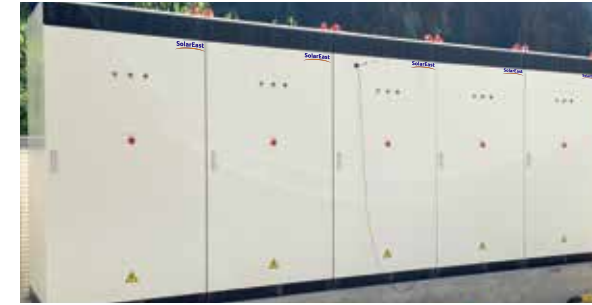
Tibet Pure Land Industrial Park Energy Storage Project
