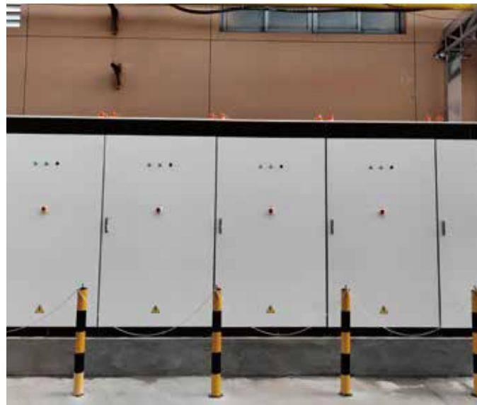
Zhejiang Textile Factory Energy Storage Project
